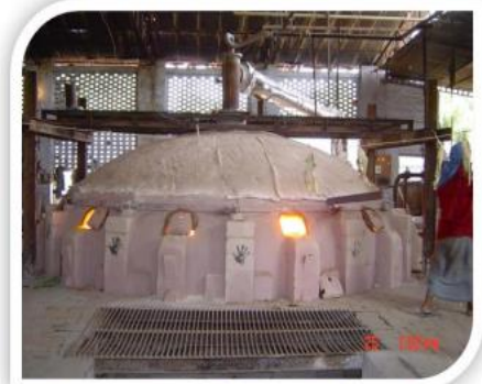
Recuperative natural gas fired pot furnace
