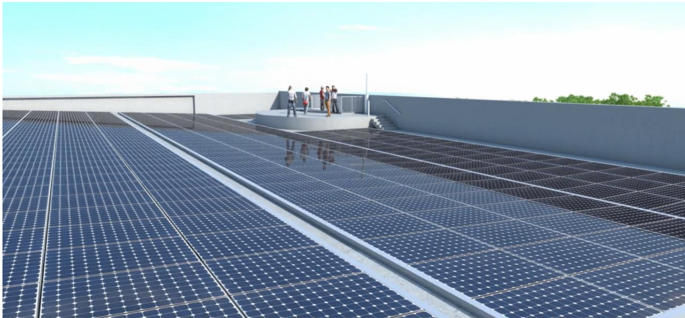
1225 PV Panels, Peak Power : 425 kWp
