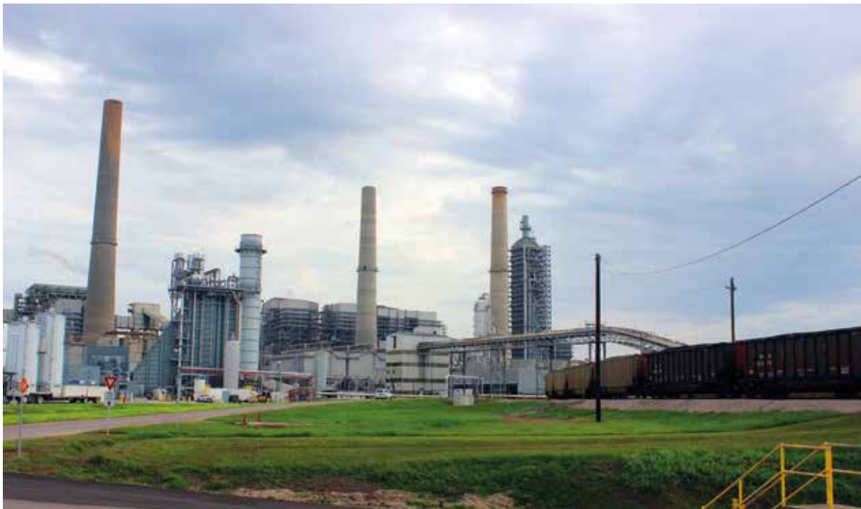
The Petra Nova carbon-capture system, including co-generation unit (left), at the WA Parish generating station (coal-fuelled units 6, 7 and 8 visible behind the system). (Image credit: NRG)
