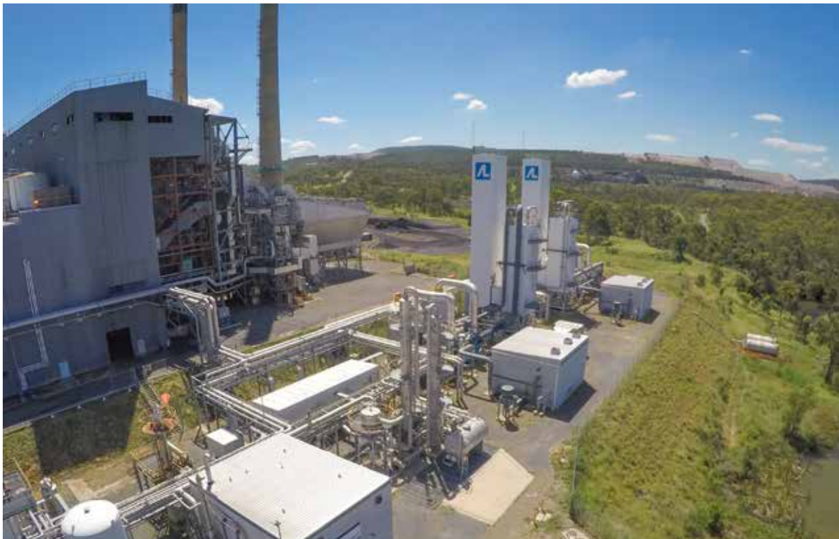
Air separation units and associated pipes and vessels at the Callide oxyfuel plant, Queensland, Australia (Image Credit: Callide Oxyfuel Project)
