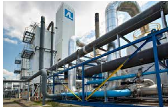
An aerial view of the Callide oxyfuel plant, Queensland, Australia (Image Credit: Callide Oxyfuel Project)
