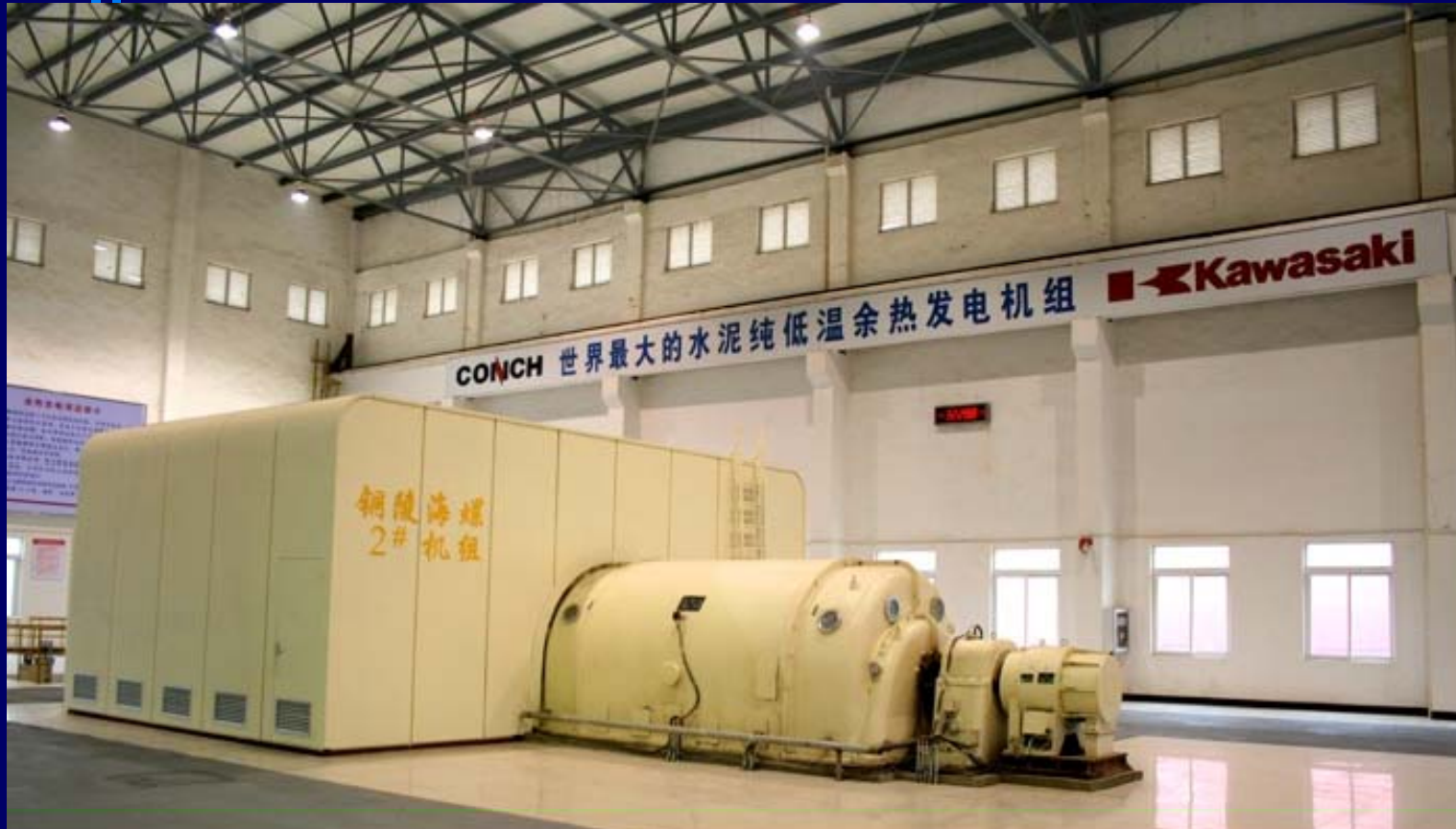
Tongling Conch Residual Heat Power Generator 2# (30500kW)
