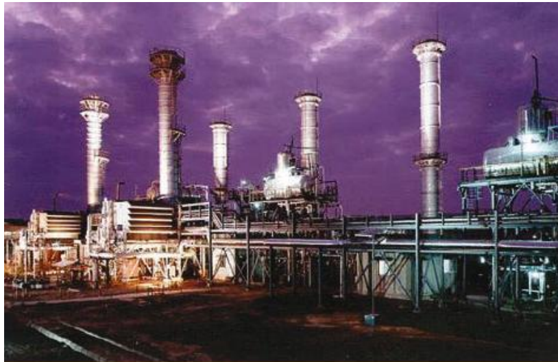
CHP Plant: Arvind Textile Mill, India
