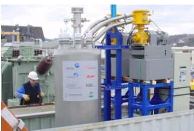
Distribution Voltage Fault Current Limiter demonstrated successfully by the EC-funded CURLIO project.
