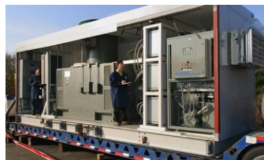
HTS enables smaller, lighter, more efficient rotating machines (motors, generators and synchronous compensators) with hitherto unattainable performance. After years of tests, TVA ordered several of AMSC's SuperVar machines to increase the stability and power quality on TVA's system.
