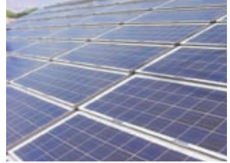
On-site renewables is an important contributor to energy security and emissions reduction (Schott Solar)
